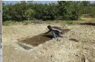
Reedbed preparation to clean Shower waste water
